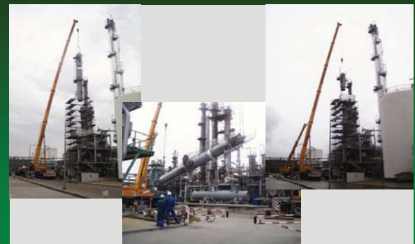
Krupp Uhde Implementation of the Ruhr Oel (Veba) Mönchsmünster Benzene Removal Project
